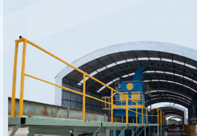
Shot Blasting & Painting Facilities
